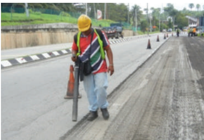
Compressed air blower
